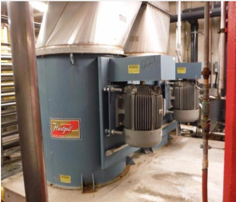
Exhaust fans of semiconductor factory
